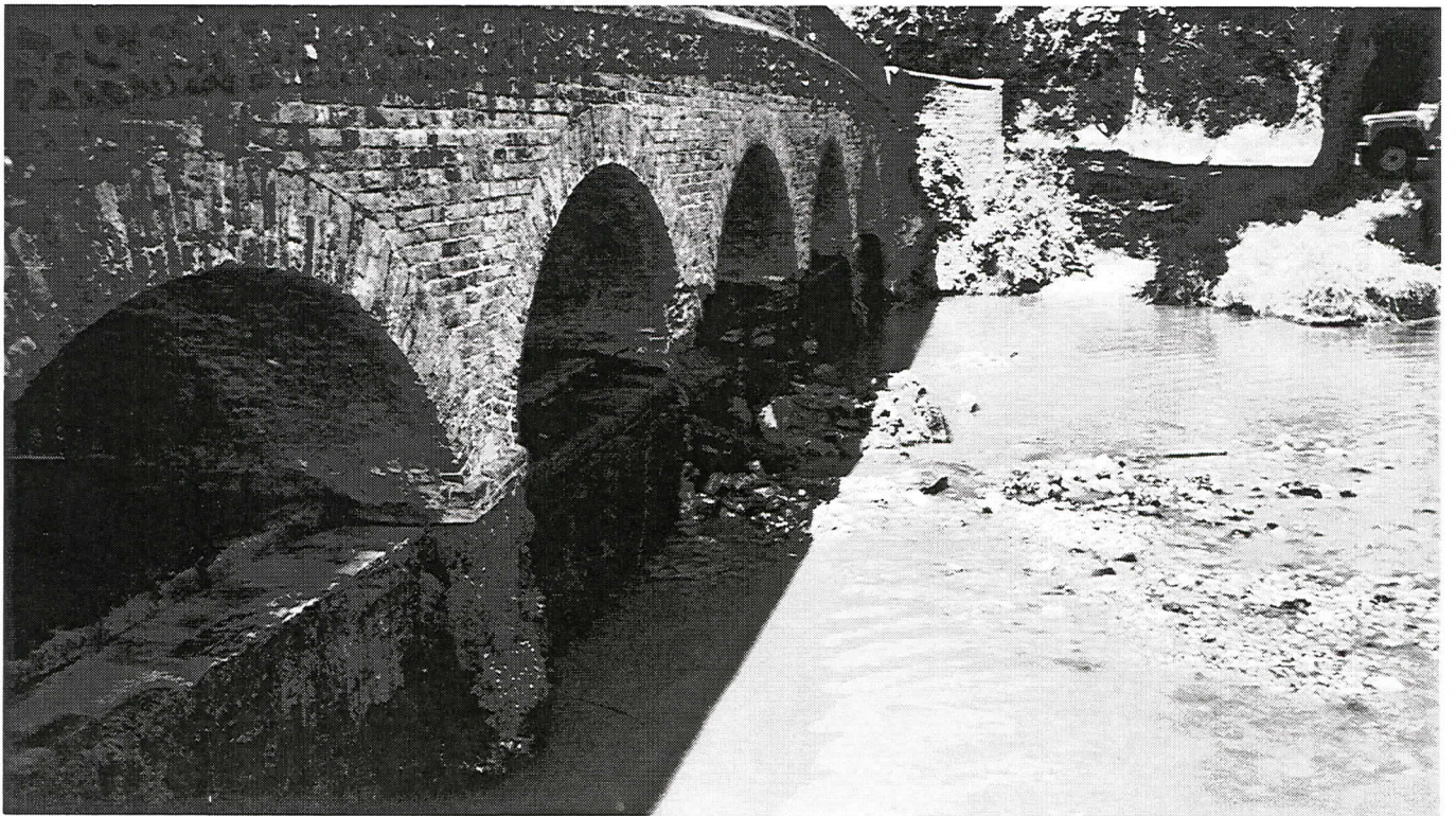
Devastation at Five Arches Bridge, Footscray Meadows July, 2001
